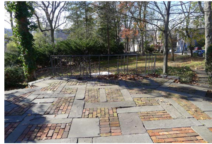
C Existing guardrail does not meet code
