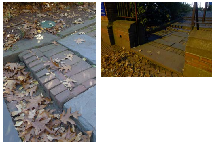
K Small uneven stairs pose tripping hazard. Too steep at top.
