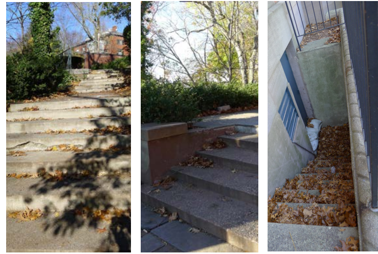
B+G+L Stairs do not have handrails.
