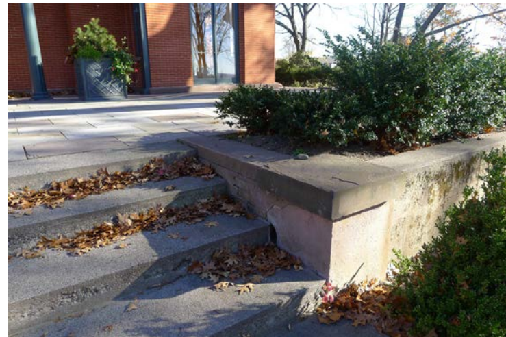
J Cheek walls on both sides of stair cracked.
