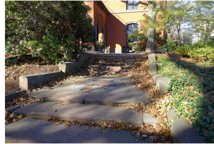
3 Blocked sight lines create dangerous hiding areas.
