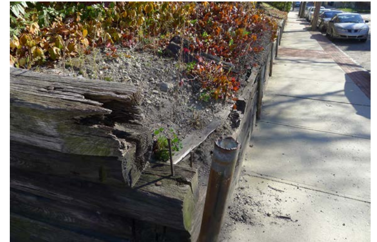
H Timber wall in poor condition. Steel posts cause safety hazard.
