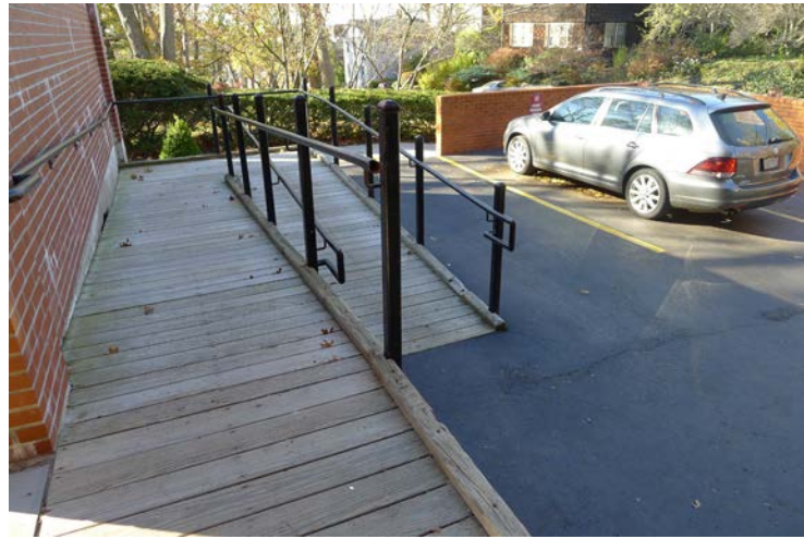
A Handicap Ramp not ADA compliant
