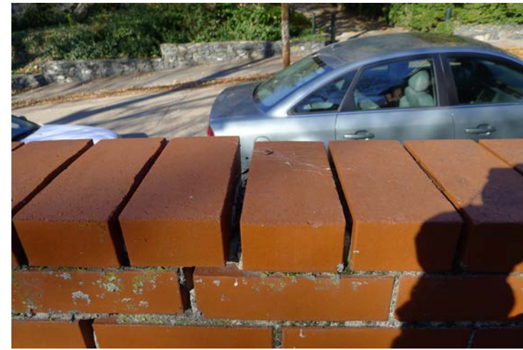
G Eroded mortar on cap
