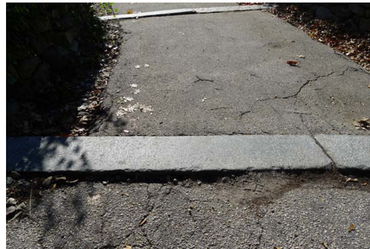
F Asphalt is sunken against granite
