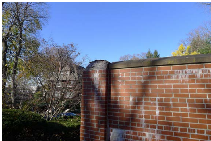
I Pillar cap eroded
