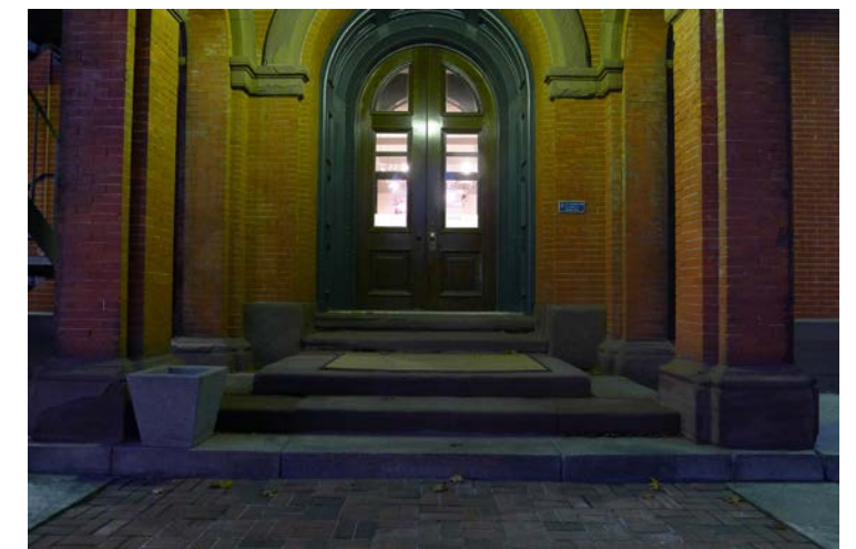
I Entry stairs are uneven
