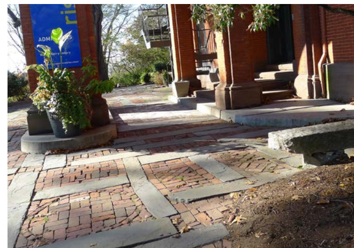
H Bluestone and brick paving is uneven
