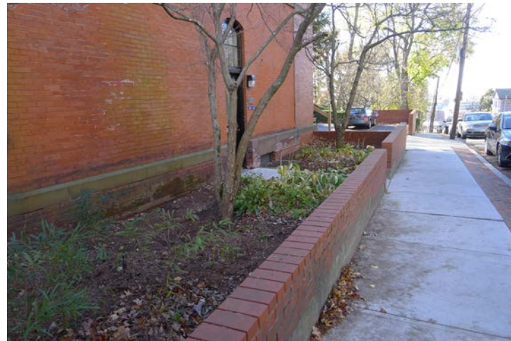
K Moss needs to be cleaned off wall and repointing as needed.
