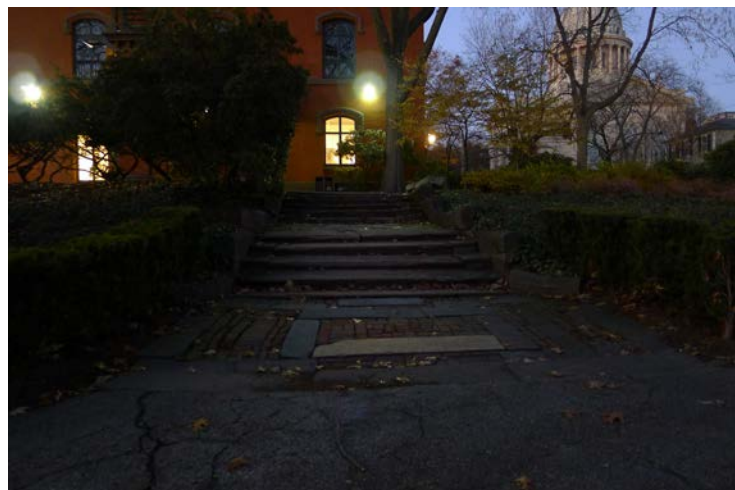
G No lighting on stairs.
