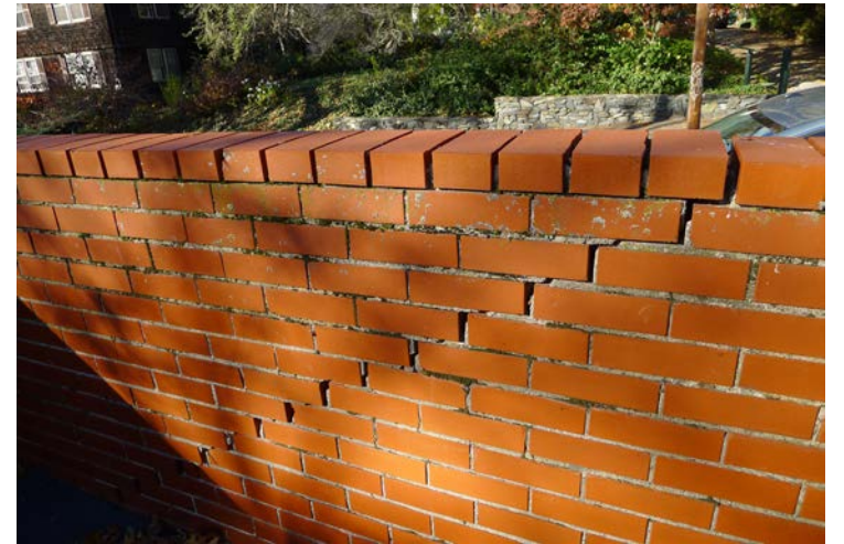
H Cracks in brick wall
